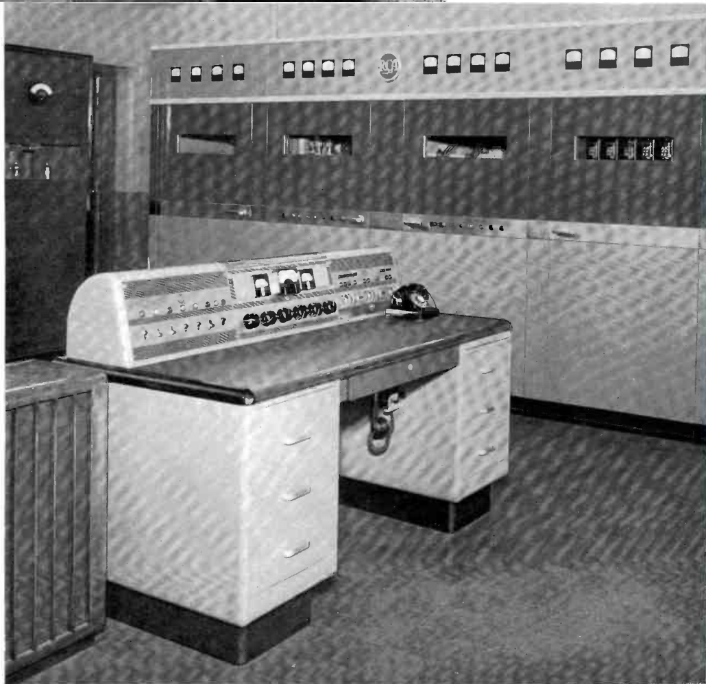
(Right): Transmitter Room in WMC's plant located on Thomas Road, 12 miles east of Memphis. New RCA 10-F Transmitter (right), the 10-F Control Console (center) and a corner of the 500-watt auxiliary transmitter (left) are shown. Audio, monitoring, and test equipment are on a rack to the right of the 10-F and are not visible in this view.
